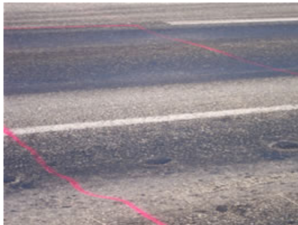
Leveling course for Tudor Road; Anchorage, Alaska. Photo courtesy of Mohammed Javed Ahmed.
