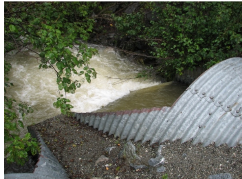
Eska Creek Culvert in need of improvements to allow for better fish passage. Photo Credit: Brian Winnestaffer, Chickaloon Village
