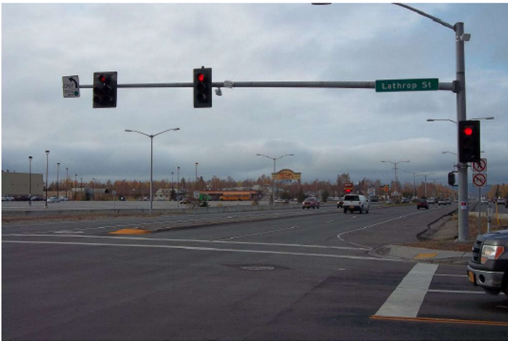
Complete radar detector installation at Lathrop St & Airport Way, facing west. The detector immediately to the right of the center signal housing is the stop bar detection for eastbound traffic. The second detector to right of the center signal housing is the advance detector for westbound traffic. Proper orientation of detectors and appropriately identifying approach speeds and line of sight at each intersection leg is critical for the initial setup of radar detection.
