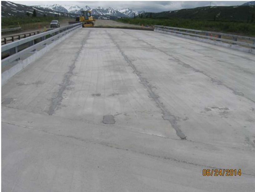
Figure 1: “A 3 part primer (2 parts with a hardener) was rolled onto the deck. There is a 12 minute gel time once the hardener is added so this process was done by mixing a single 5 gallon bucket at a time. This process took approximately 1 hour.”
