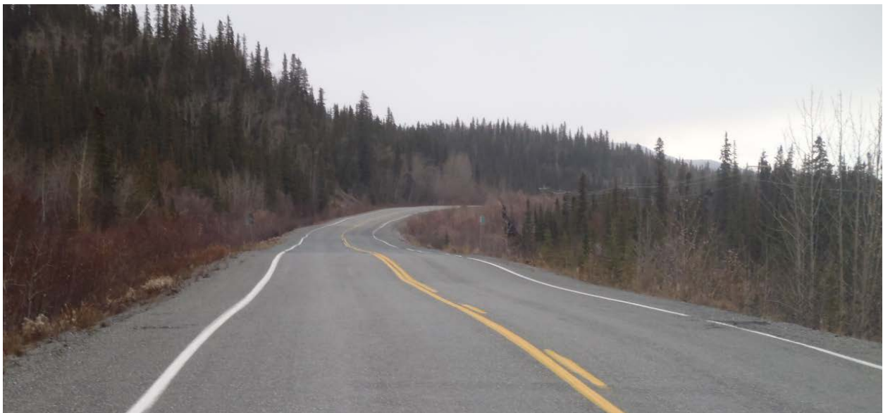
Exhibit 3. Soil slope in Poor condition, Tok Highway. Movement is relatively rapid, necessitating frequent maintenance to keep the road passable.
