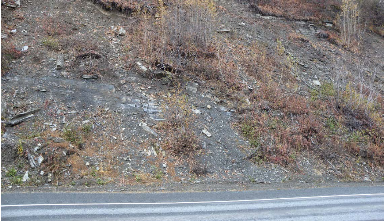
Exhibit 2. Rock slope in fair condition, South Tongass Highway. Rockfalls are occasionally able to reach the road and cause a safety hazard.
