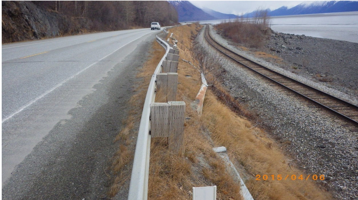
Exhibit 4. Retaining wall in Poor condition, Seward Highway. The wall is bowed outward, causing deformation of the guardrail and pavement (which was recently repaired but is already cracking again).
