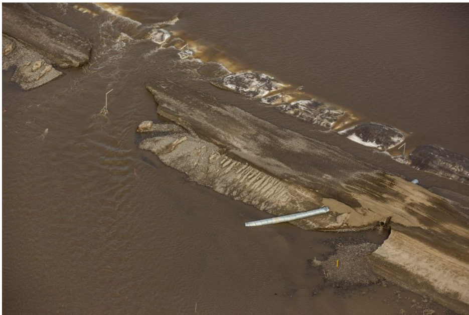
Exhibit 10. April 2015 washout of the Dalton Highway due to unusual North Slope spring break-up conditions
