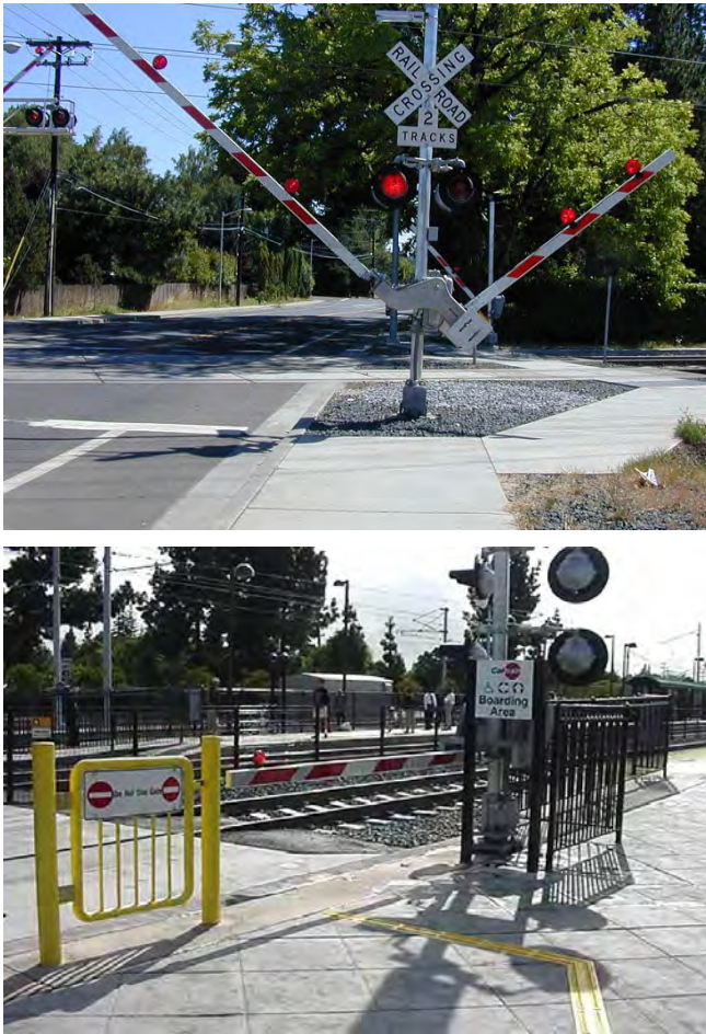
Figure 76. Pedestrian Automatic Gate Examples
