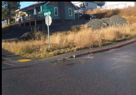
Flooded and Icy Curb Ramps
