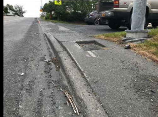
Settled Electrical Junction Boxes
