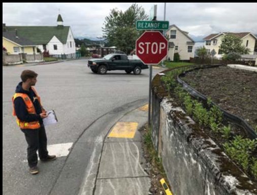
Damaged Retaining Walls Restricting Sidewalk Space
