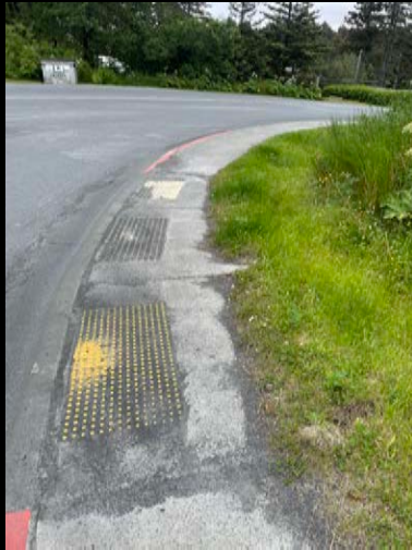
Non-ADA Compliant Curb Ramps
