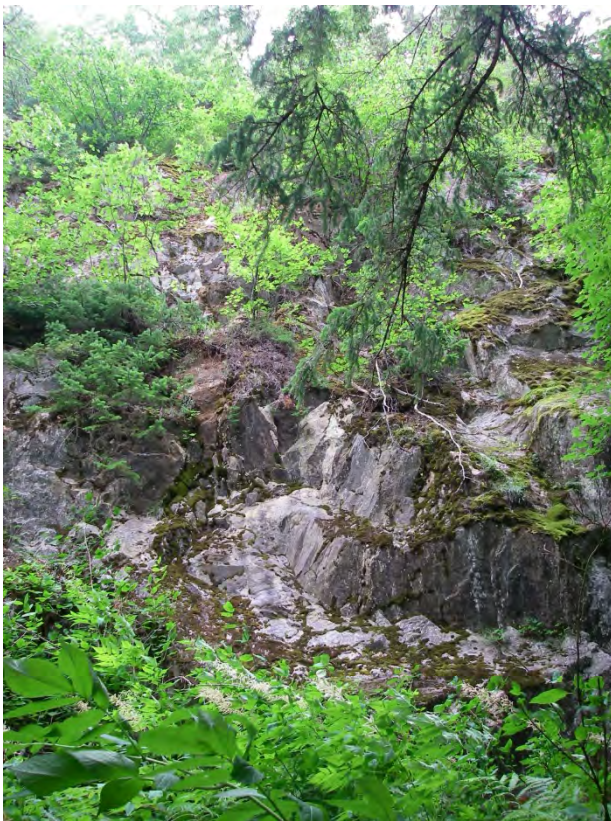
RF42. View east/upslope at rockfall hazard.
