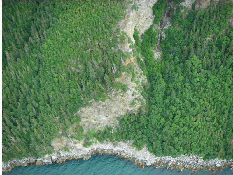
RF07. View east/upslope at 500 ft high gneiss cliffs with strong jointing and rockfall.
