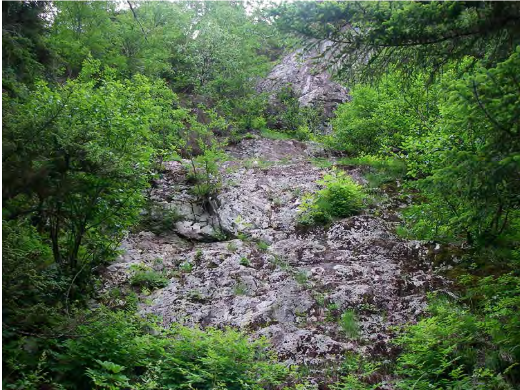
RF01. Basalt cliff that is the origin of rockfall hazard.
