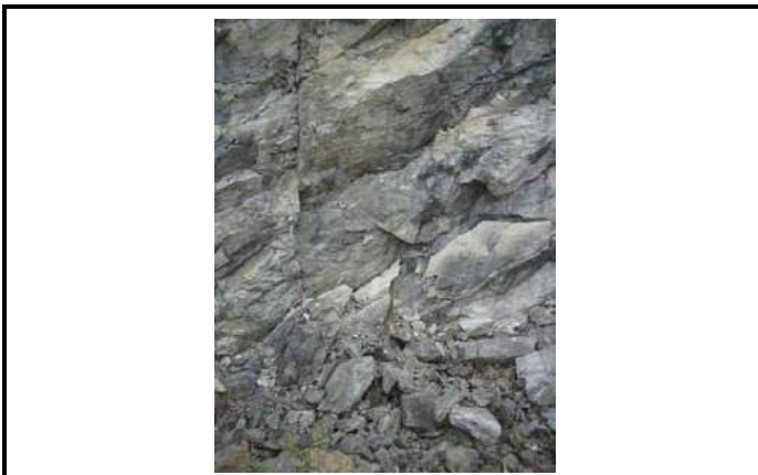
Cut on Road to Community Water Supply
