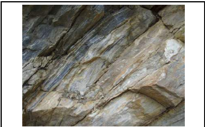
Cut on Road to Community Water Supply
