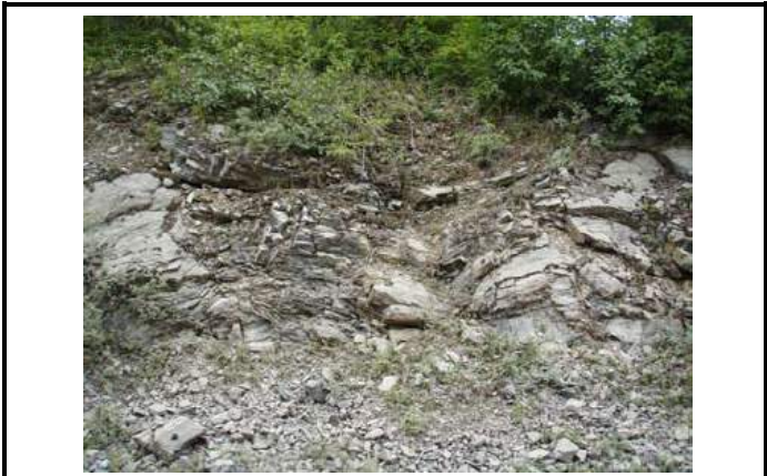
Cut on Road to Community Water Supply
