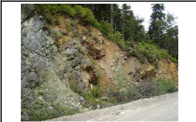
Cut on Road to Community Water Supply
