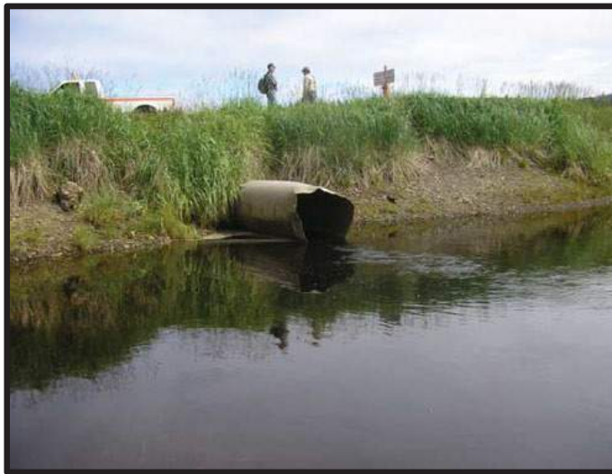
Photo 9- Shotter Creek perched undersized culvert.
