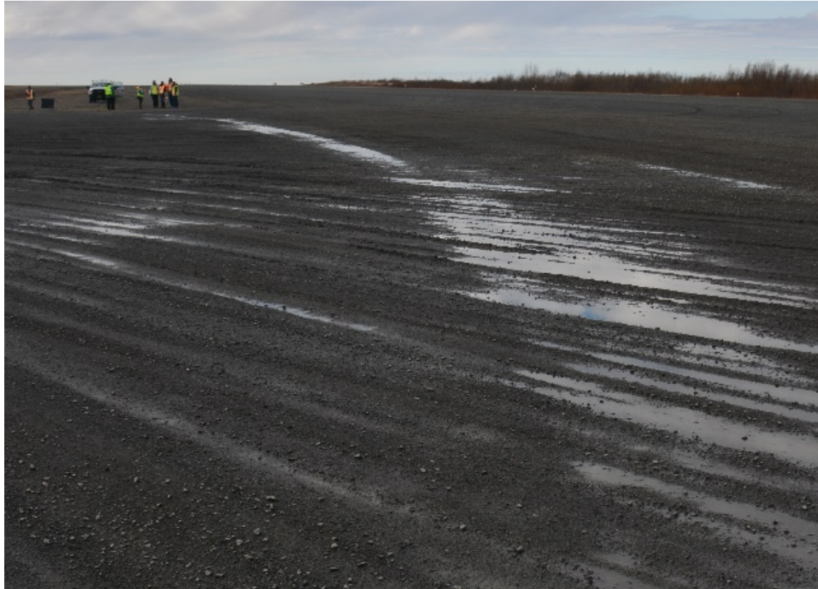
Graphic 2: Current Taxiway B Surface
