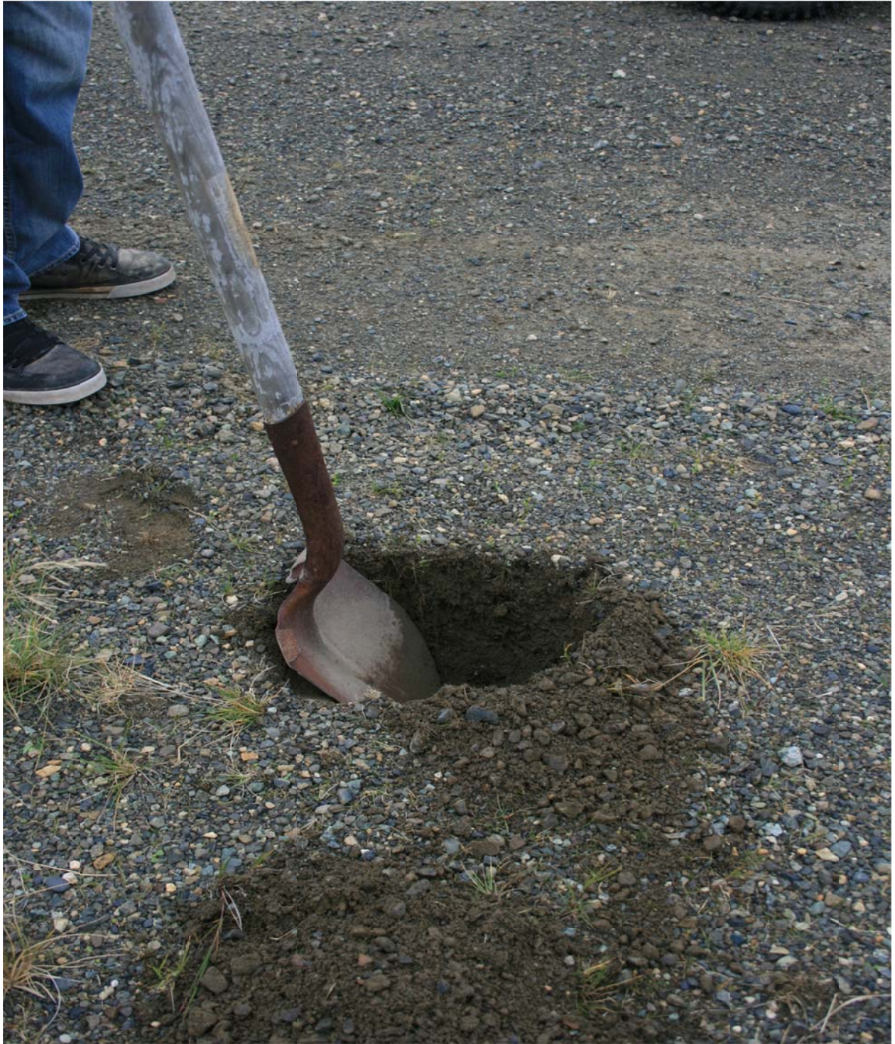
Figure 4: Hole on side of the runway showing a shallow depth of gravel
